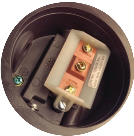
Figure R-5 DP-1A Terminal Block
