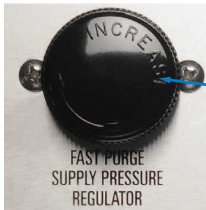
Figure F-11 Fast Purge Supply Pressure Regulator
