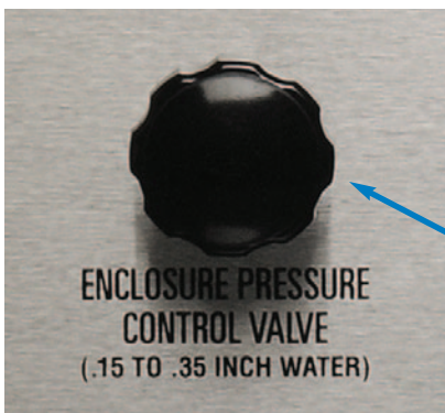
Figure F-16 Enclosure Pressure Control Valve
