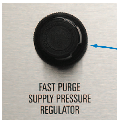
Figure F-11 Fast Purge Supply Pressure Regulator
